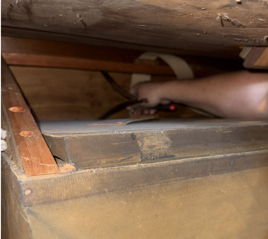
Jim Griesemer had a tough reach to remove the broken strap and replace it with a new one.
