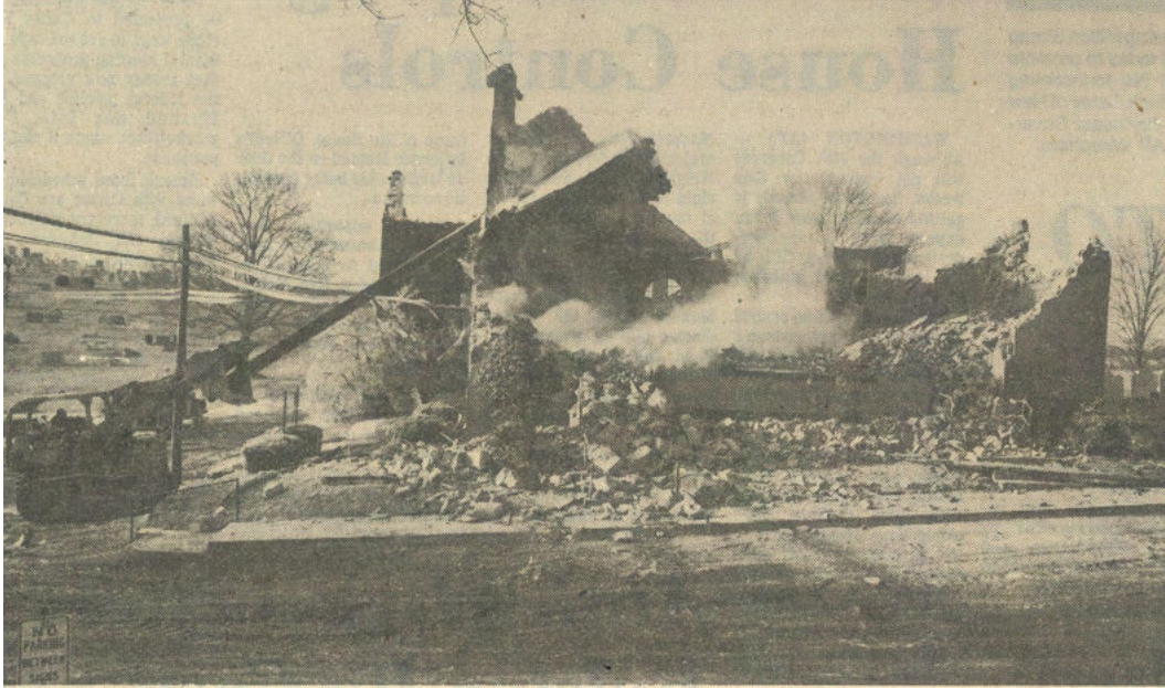
MODERN DAY BUGLES — The walls of historic St. Daniel's (Corner) Lutheran Church in Heidelberg Township came tumbling down Wednesday afternoon, but congregation members are reading plans to build a new church. The trees and bushes surrounding the church are still covered with ice from the water firemen used to extinguish the four-hour blaze Wednesday morning at the church.
