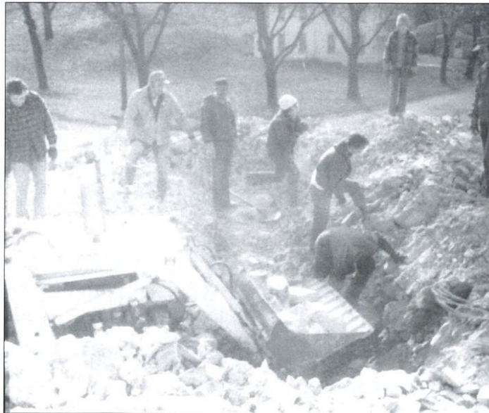
Members sift through the rubble.
